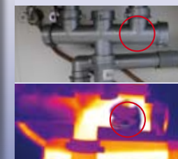
The blockage in this pipe is quickly located using a thermal camera. Action will be taken before the problem worsens.
